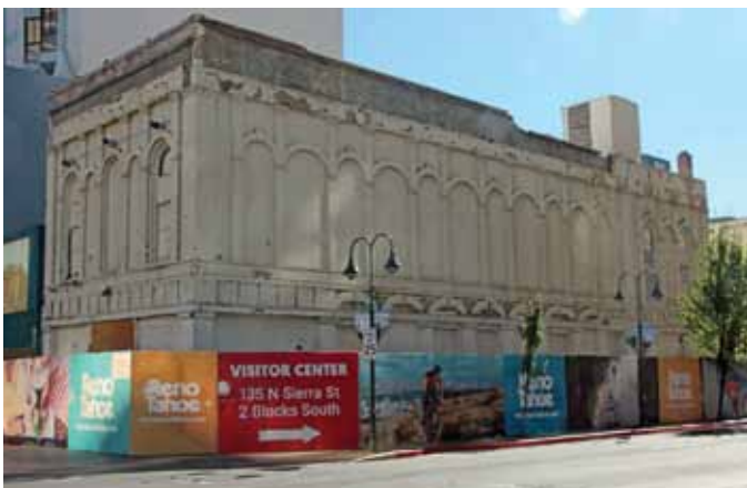
The Masonic building at Commercial Sierra in October 2018, fenced off and awaiting demolition. Courtesy David Lowndes.
