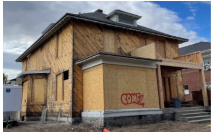
September 2025, this lovely building appeared to be under construction? Or wrapped in plywood? Courtesy Debbie Hinman.
