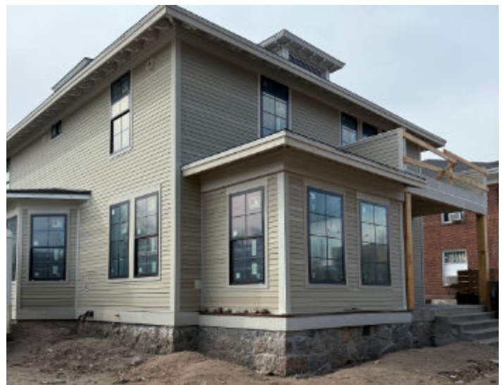
Unveiling the building under the plywood that has been replaced with new shiplap siding, echoing the building’s original appearance. Note the dormer atop the house with its original window. Courtesy Debbie Hinman.
